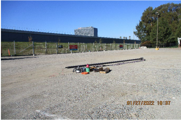
Photo 1 - 25th N Yard Lighting Pole
