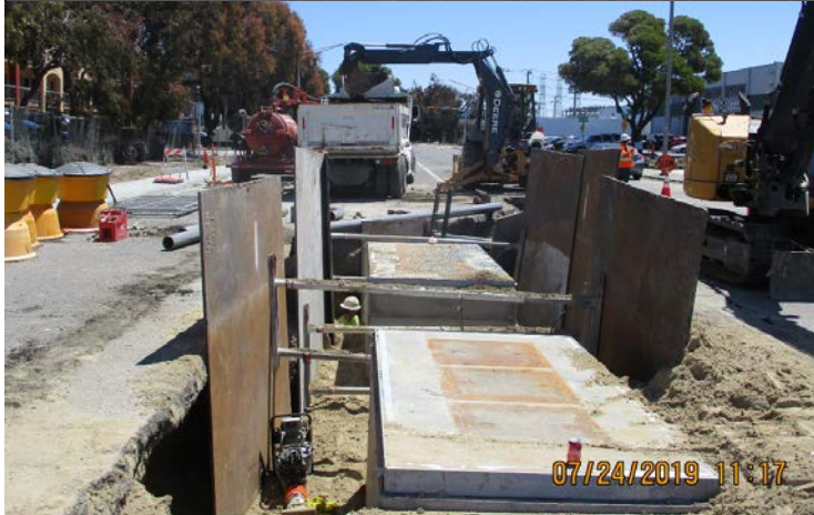
Splice boxes on Grand Avenue
