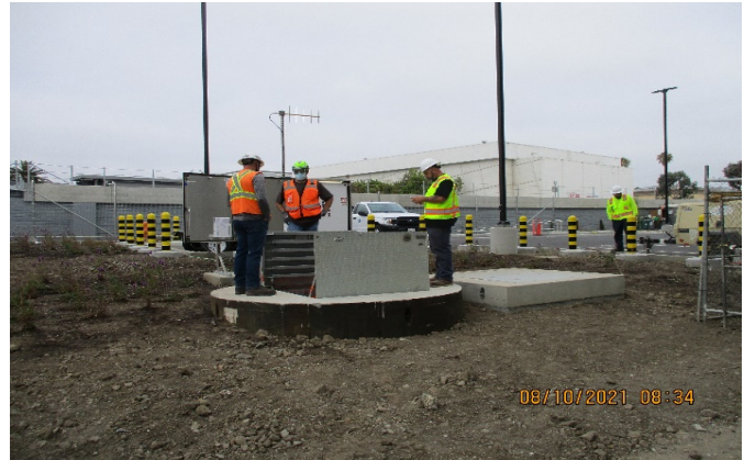
Photo 2 - Pump Station Testing
